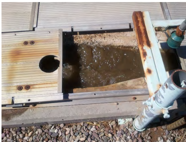
Parshall Flume at Headworks
