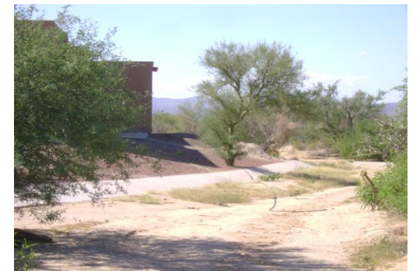
Elevated Home with concrete scour protection In all cases scour protection shall be designed to be a minimum of three feet below the lowest point of the adjacent channel thalweg.
